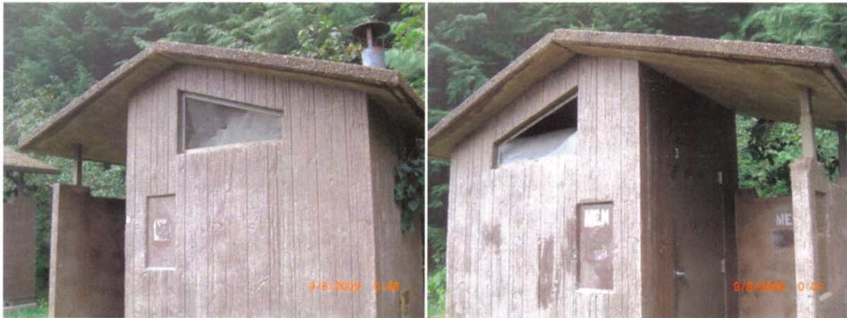
Figure 2. Two CXT-type outhouses at the parking area have significant damage.
